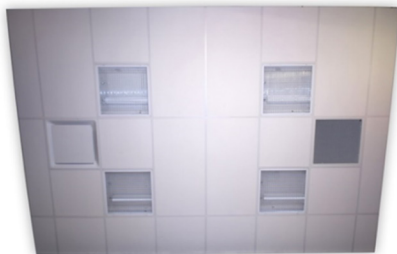
Reference ceiling with four lights (center), air diffuser (left) and return grille (right).
